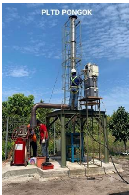
Figure 3. Enerflow Cyclone Burn Grate PLTD Pongok Source: Field Test Documentation, 2026
