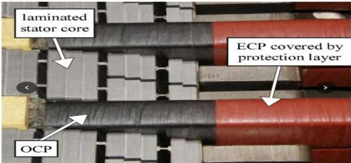
Picture 2. Coils that already use corona shield (P8003)
