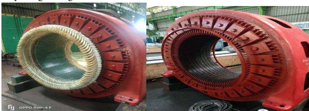
Picture 6. Condition of the stator after rewinding
