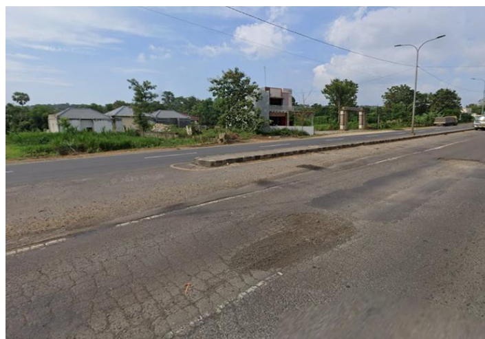
Figure 4. Documentation of cracks on the road surface Source : Field Survey,(2025)
