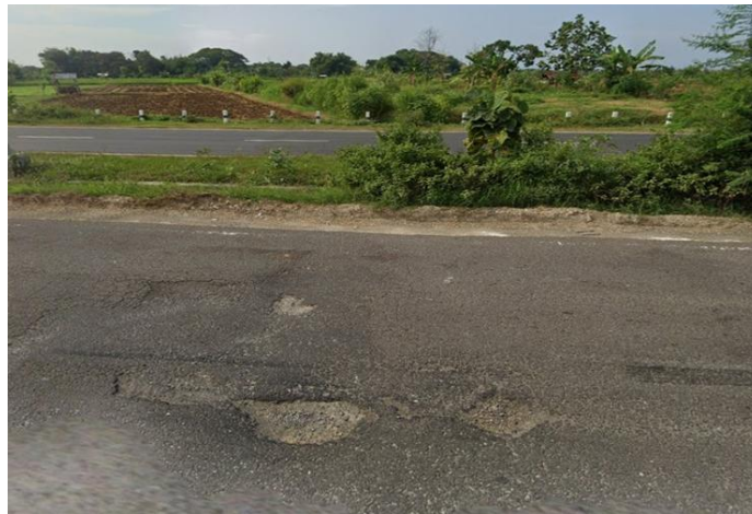
Figure 3. Pothole Road Surface Documentation Source : Field Survey,(2025)
