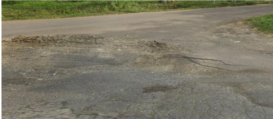
Figure 5. Documentation of the Surface of the Undulating Road Source : Field Survey,(2025)
