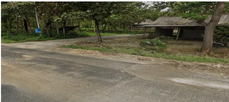
Figure 7. Uneven Patch Road Surface Documentation Source : Field Survey,(2025)
