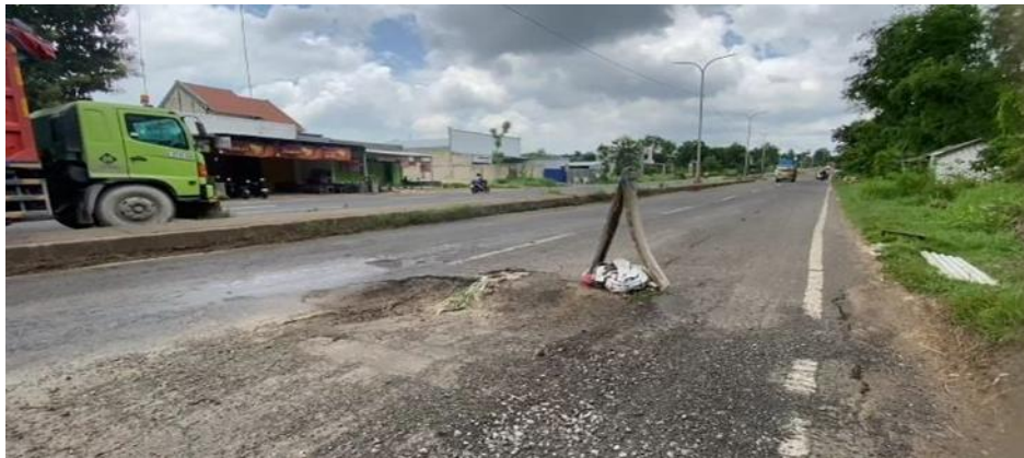
Figure 6. Documentation of the Surface of the Bumpy Road Source : Field Survey,(2025)
