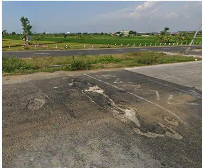
Figure 2. Documentation of potholes road surfaces Source : Field Survey,(2025)
