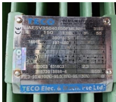
Figure 2. Photo of 110 kW Induction Motor Nameplate
