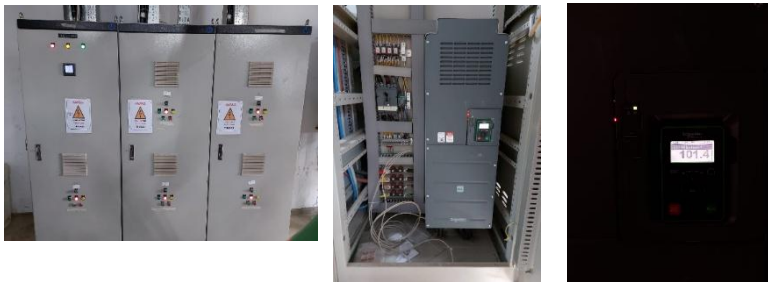
Figure 1. Photo of Schneider ATV610 110kW Inverter Panel
