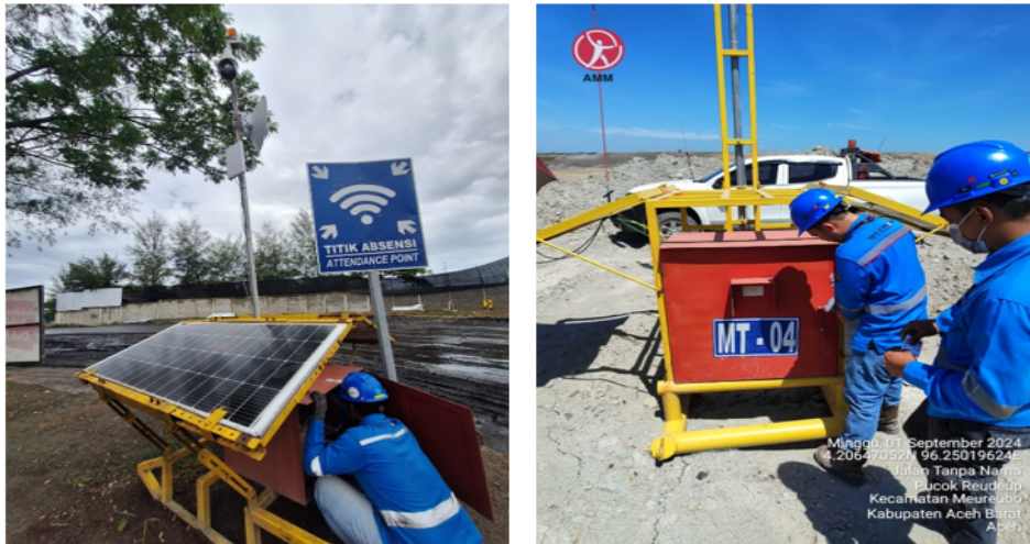
Figure 1. Mobile Tower SS6 Wifi Installation
